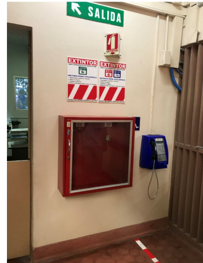
Figure 12. Missing Fire Extinguisher (By Authors)
