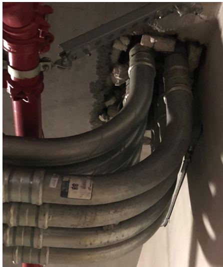
No fire stopping
